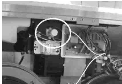
5.To replace the tube starter.
